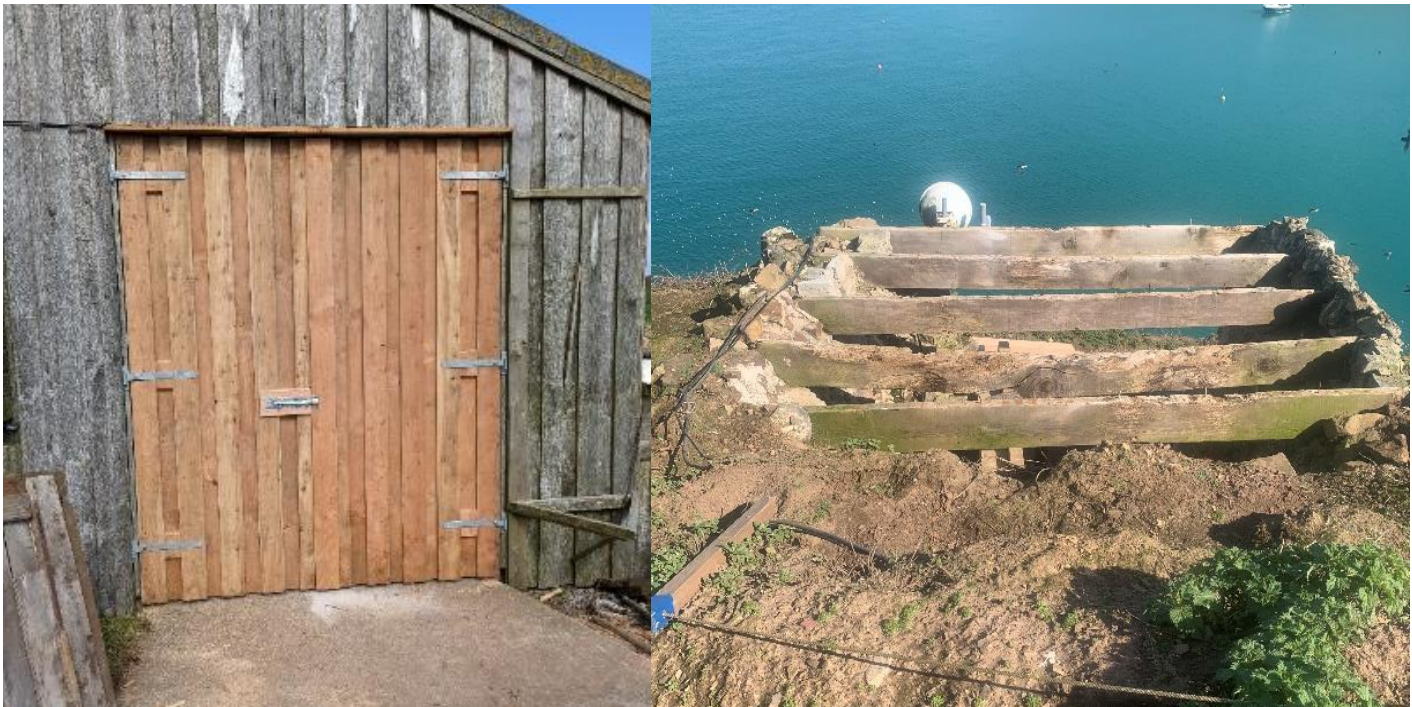
New garage doors at North Haven and the Lime Kiln roof in the process of being replaced
