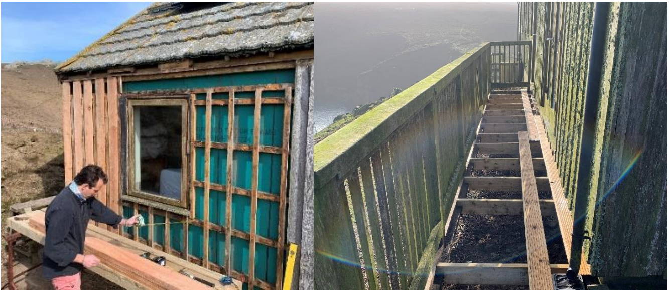
Other spring Work Party tasks of replacing cladding and repairing the research balcony at North Haven
