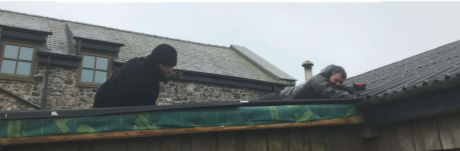
Battery Room roof replacement still in progress but in far worse weather
