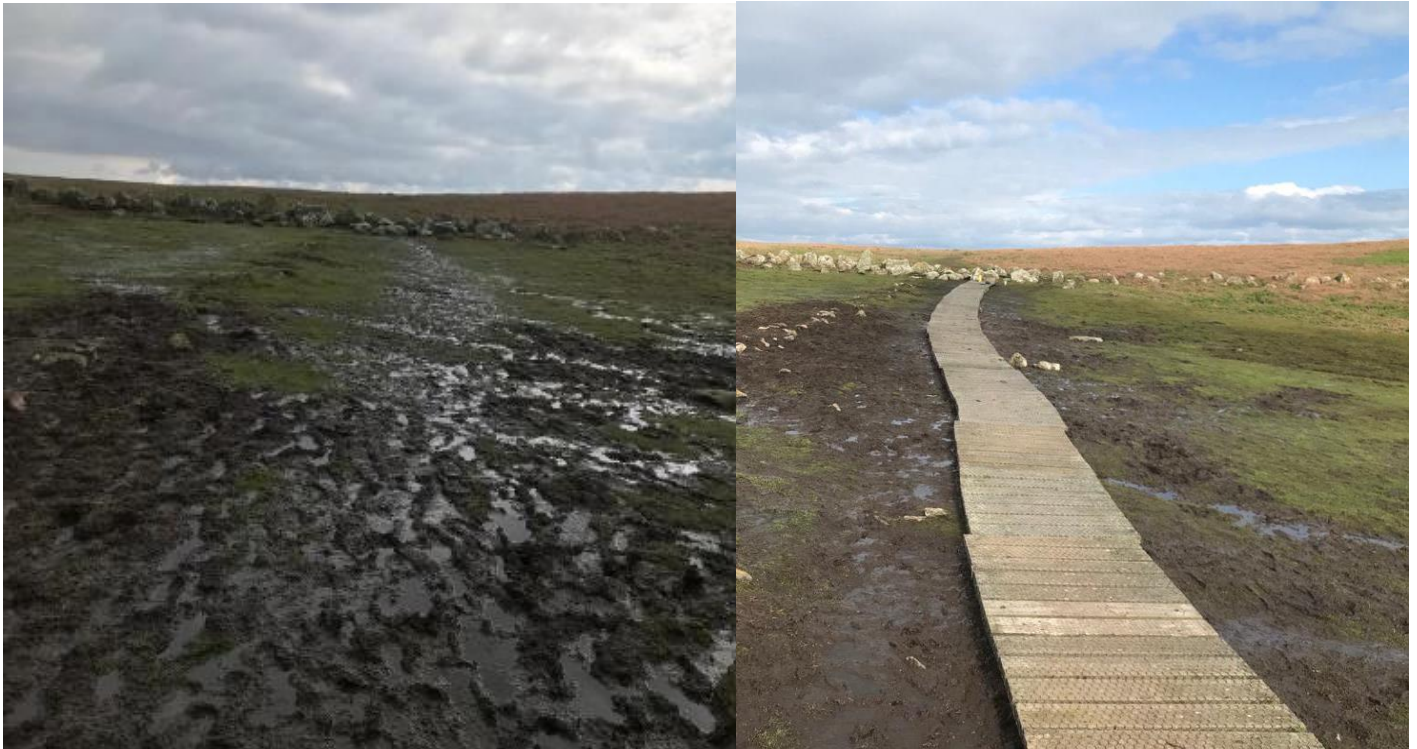
Before and after. A temporary boardwalk is placed over the wet spring flush at Tom's House to reduce poaching and widening of the paths
