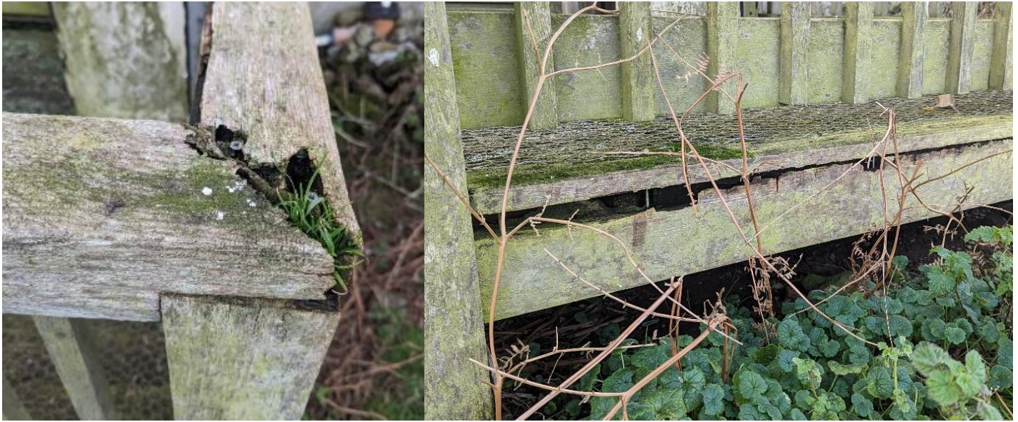
Future infrastructure work - rotting handrails and joists on North Haven balcony.
