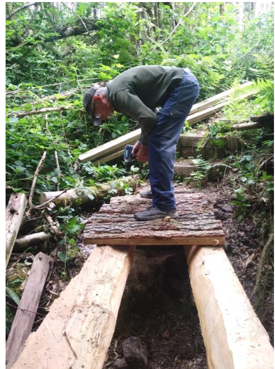
The new bridge under construction at Coed Maidie B Goddard. (Photo Doug Lloyd)
